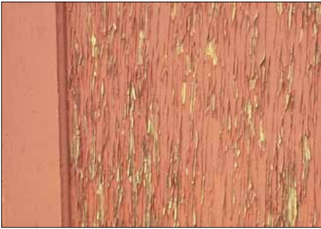
Figure 16-9. Early paint failure on plywood caused by penetration of moisture into surface face-checks.
