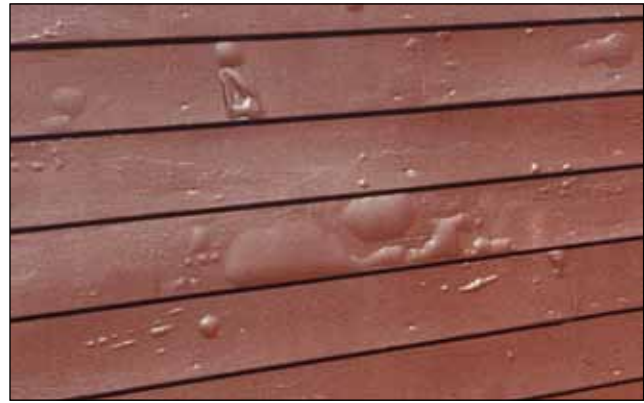
Figure 16–21. Water blisters (also called moisture blisters) caused bubble-like deformation of paint film.
